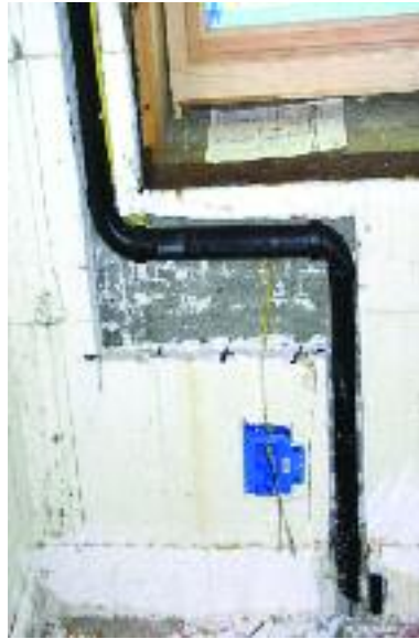
Fig 3.9 – Electrical installed in an Amvic ICF wall.
