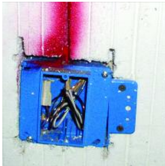
Fig. 3.8 – Electrical installed in an Amvic ICF wall.
