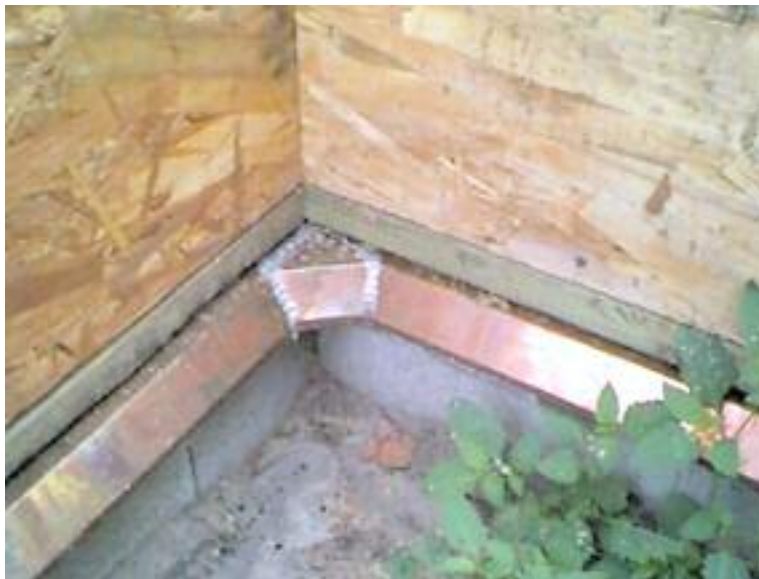
Figure 8.12 – Detail of metal shield at corner. Copyright ©1998-2005, Urban Entomology Program, University of Toronto www.utoronto.ca/forest/termite/termite.htm
