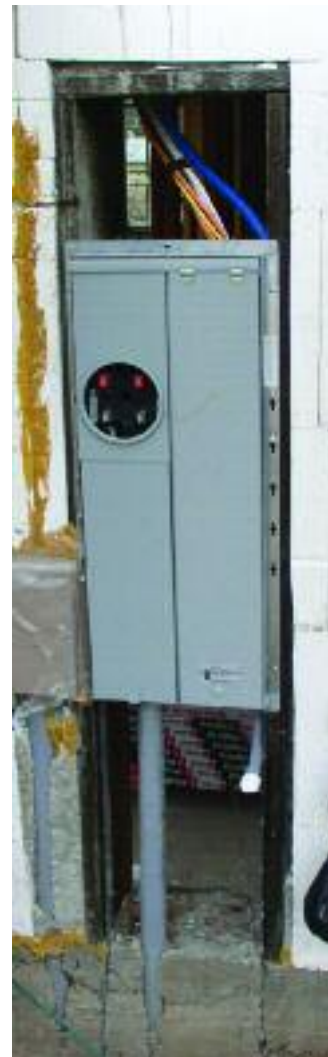
Figure 8.1 – Main electrical panel installed flush with exterior wall
