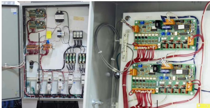
Zone Board location inside electrical cabinet.
