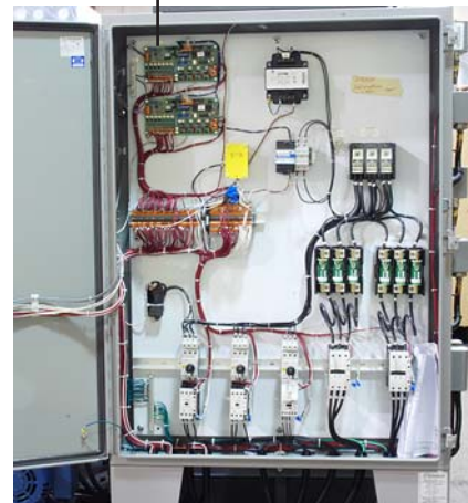
Zone Board location inside electrical cabinet.
